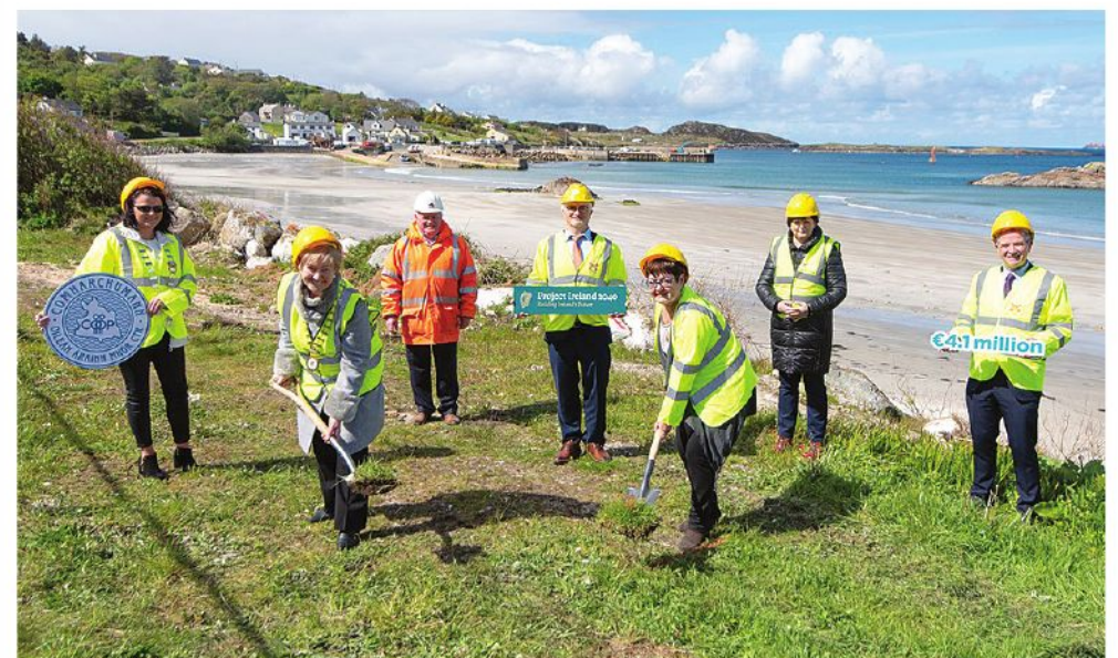
(Below): Cathaoirleach of Donegal County Council, Cllr. Rena Donaghey and Bainisteoir, Comharchumann Oileán Árann Mhór Teo, Ms. Nóirín Úimhaoldomhnaigh turning the sod on the Aranmore Island Shore Front Amenity Development. Back Row (L-R): Cllr. Marie Therese Gallagher, Cathaoirleach of the Glenties Municipal District, Joseph McMenamin, Contractor, John McLaughlin, Chief Executive of Donegal County Council, Cllr. Noreen McGarvey, Chairperson of the Islands Committee and Liam Ward, Director of Service, Community Development & Planning Services, Donegal County Council".
